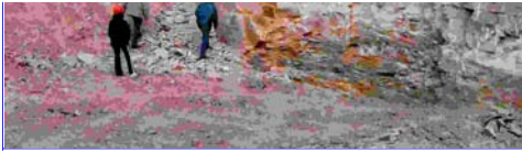
Some of the party examining the current working face in Swinton quarry. The gently dipping bedding planes can be clearly seen.
