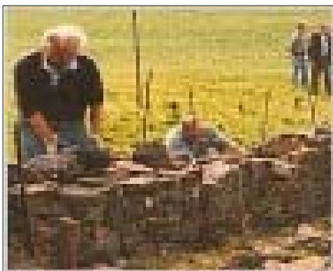
Yorkshire - Standard Wall Construction Courtesy of the Dry Stone Walling Association of Great Britain
