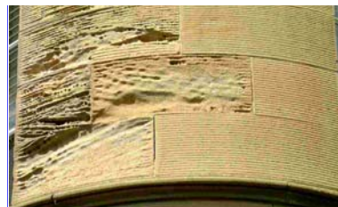
The stone on the left is original and shows honeycomb weathering. The new stone on the right is Springwell. Tooling on the replacement stone matches the original.
