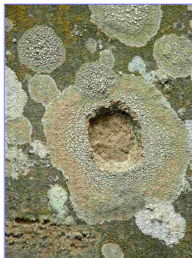
Pitting occurs in the central zone of lichen growth and may be as much as 10mm in depth.
